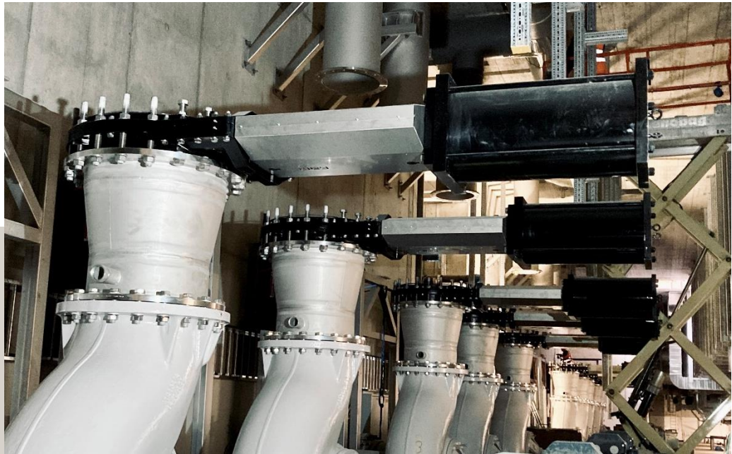
Wey MFC DN 700 knife gate valves during construction in the biological treatment unit
