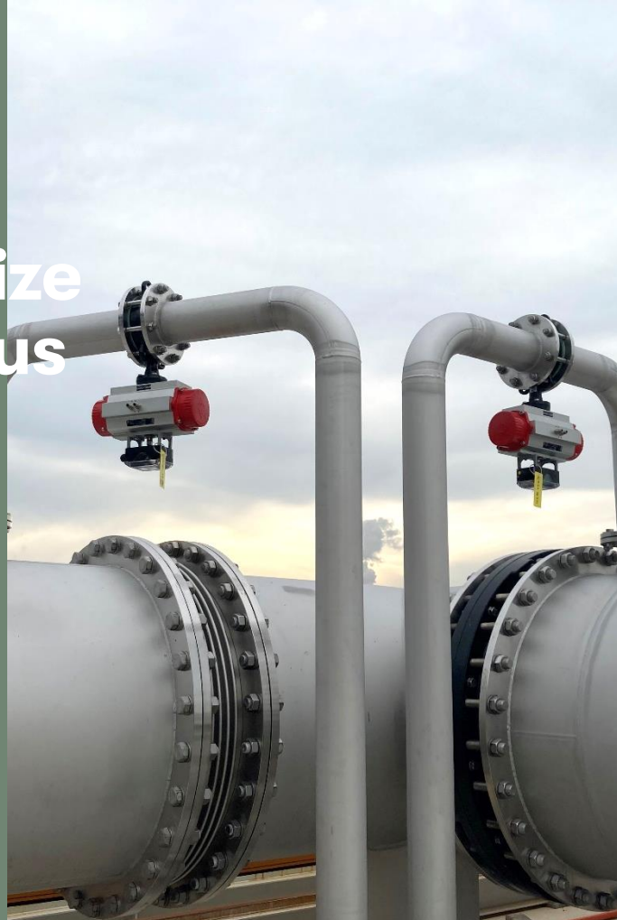
Two TW20-6 DN 125 butterfly valves on the roof of the new building
