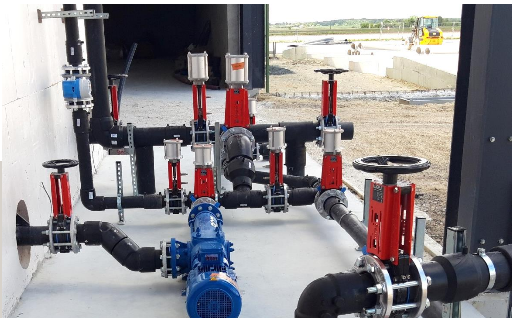
Ring installation for the distribution of the liquid digestate
